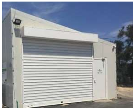
Picture 11. Automatic mechanisms in the doors
