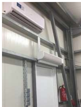
Picture 9. Two air curtains have been added in the doors of the pretreatment unit
