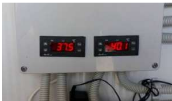
Picture 5. Temperature indication for both solar drying halls
