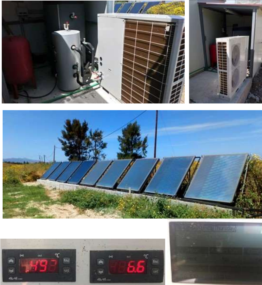
Picture 8. The heating pump and 4 more new solar panels
